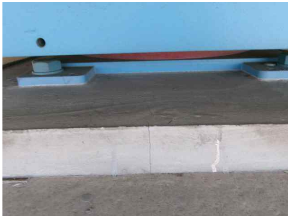
P2-Sh3 받침몰탈 균열 (0.2mm/0.2m)
